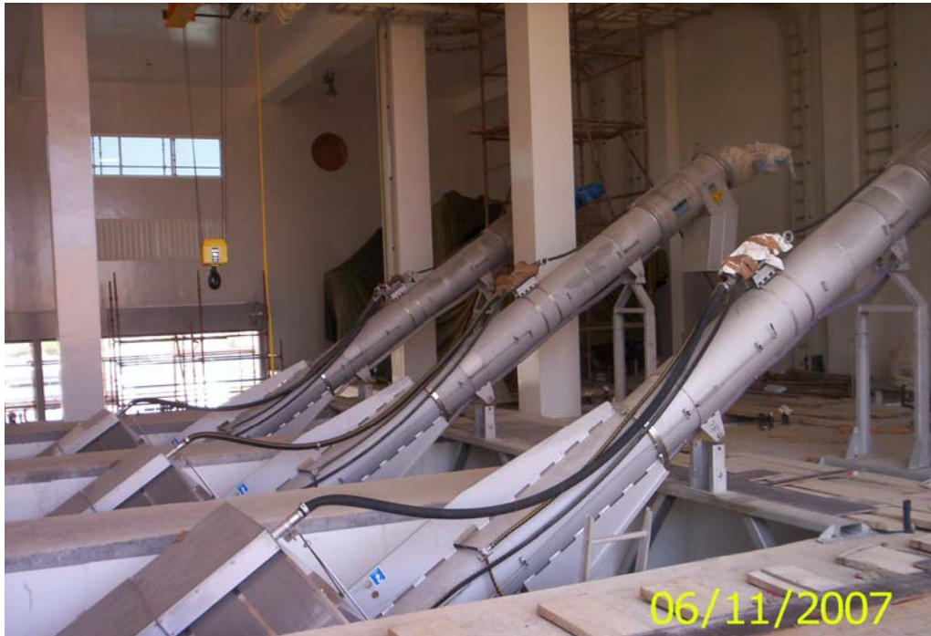
Fig.6 Al Ansab MBR – Wastewater Sieving
