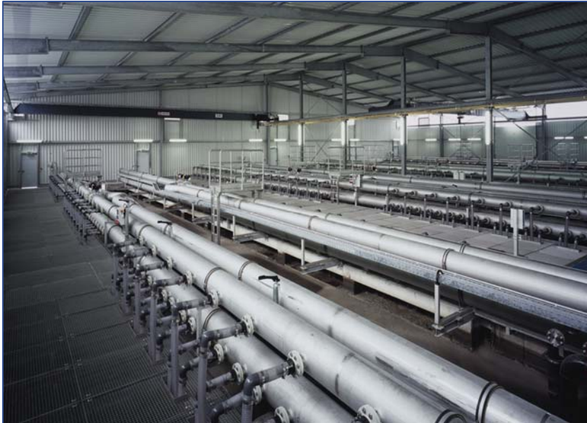
Fig.2 Nordkanal MBR – Membrane Scouring and Permeate Pipes
