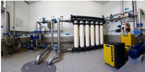
BLGACH spring water treatment plant
