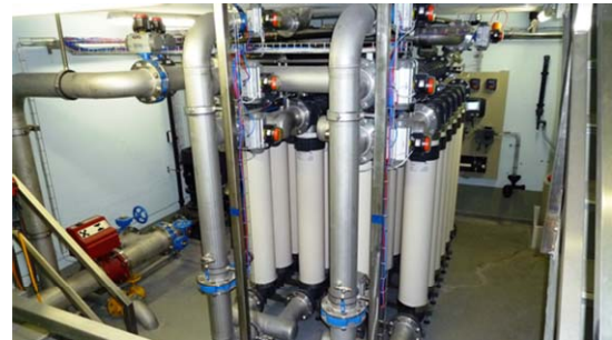
MAIENFELD spring water treatment plant
